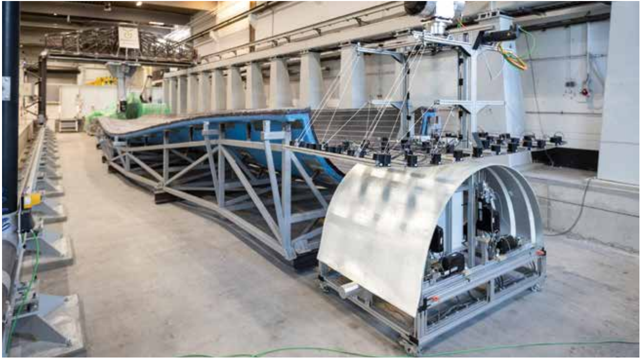
Layup of pre-cut glass fiber fabrics on a positive mold to pre-manufacture the root insert. (Courtesy: Fraunhofer IWES, Jan Meier)
