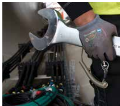
East Anglia ONE will be the first wind farm project to use 66kV cables on a commercial scale. (Courtesy: Global Wind Service)
