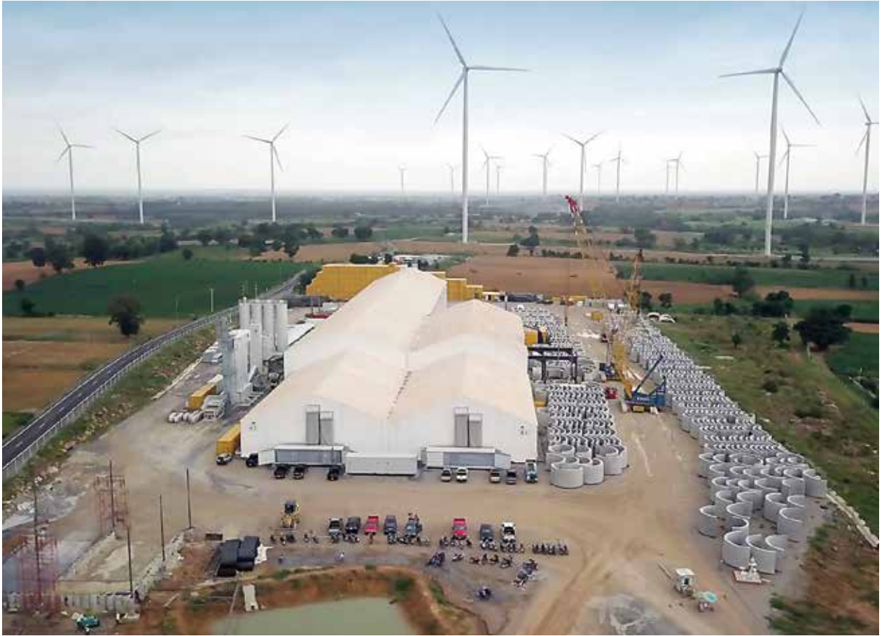
The ability to produce tower segments on site can tackle transportation challenges and aid in local job creation. (Courtesy: Max Bögl Wind AG)
