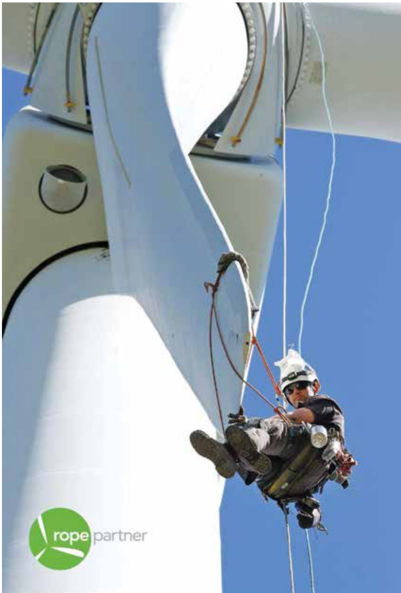
Rope Partner is recognized internationally as the premier at height service provider of repair, maintenance, and performance-enhancing services for wind-turbine blades. (Courtesy: Rope Partner)
