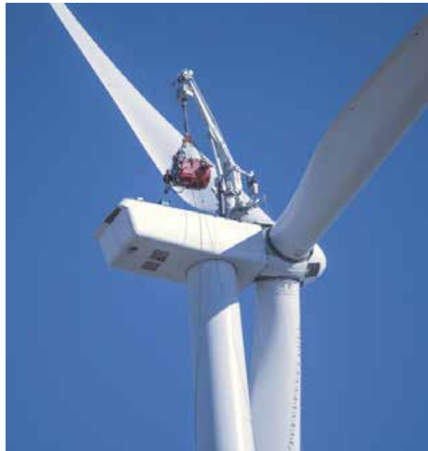
A Liftra Self-Hoisting Crane® in action. Newer, self-hoisting systems can do jobs for much less than a traditional crane. (Courtesy: Gearbox Express)
