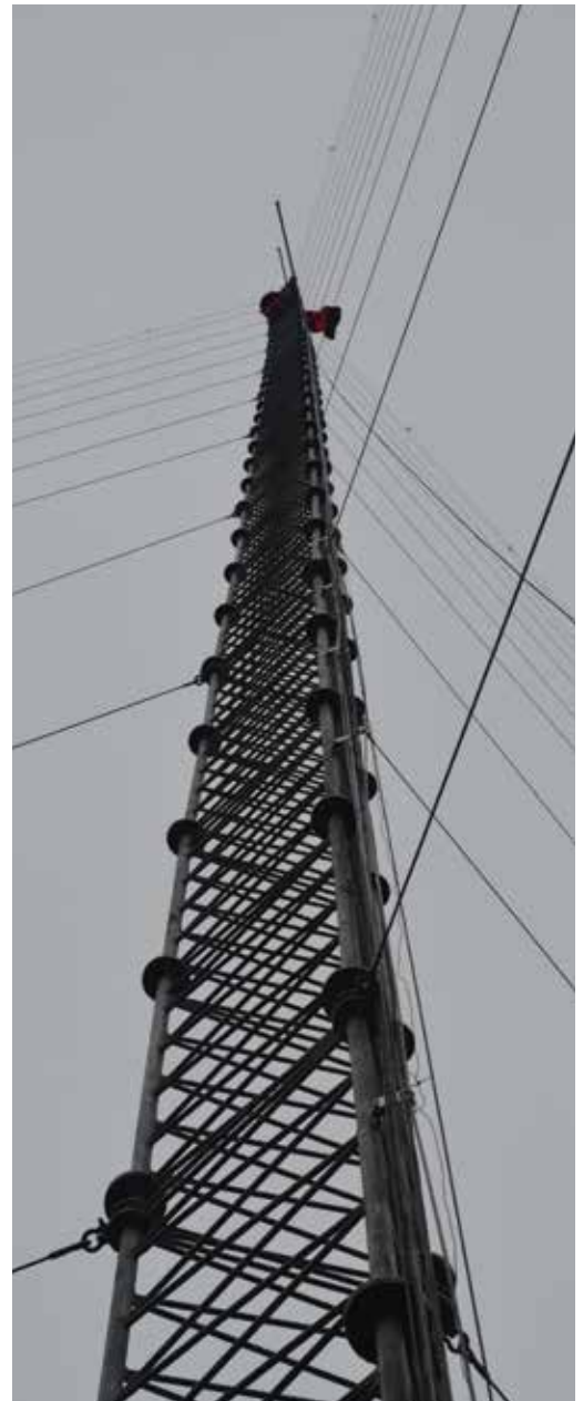
The 100-meter guyed lattice mast will provide measurement data for a major post-subsidy project in the southwest of Scotland. (Courtesy: Dulas)
