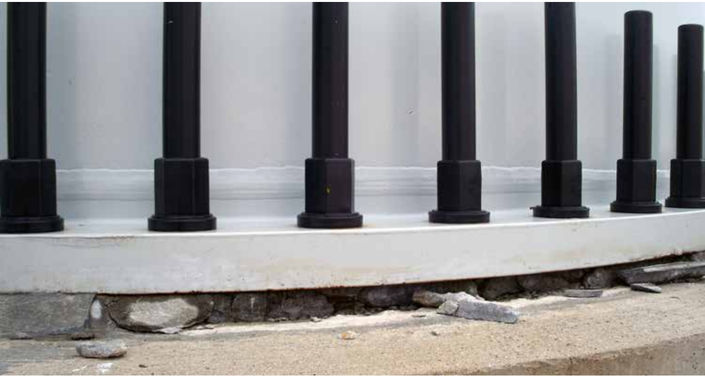
A grout failure requiring repair. (Courtesy: Wind Secure Inc.)
