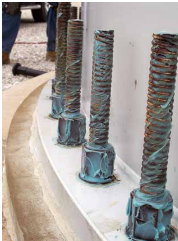
Properly greased anchor bolts ensure all exposed surfaces are adequately coated, with extra attention given to the washers and nuts where the hardware is most susceptible to corrosion. (Courtesy: Wind Secure Inc.)
