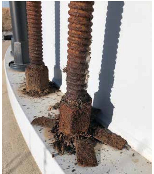
Corrosion of the anchoring hardware can lead to significant and unexpected costs to fix and jeopardize the integrity of the foundation. (Courtesy: Wind Secure Inc.)
