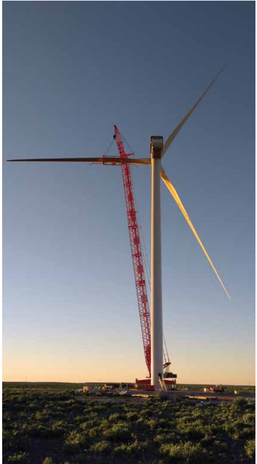
ALE providing the crane lifting and electro-mechanical installation at Garayalde, Argentina. (Courtesy: ALE)
