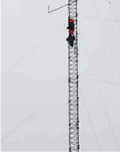
The bulk of the Dulas' work in 2018 came from meteorological mast installation, refurbishment, and decommissioning. (Courtesy: Dulas)
