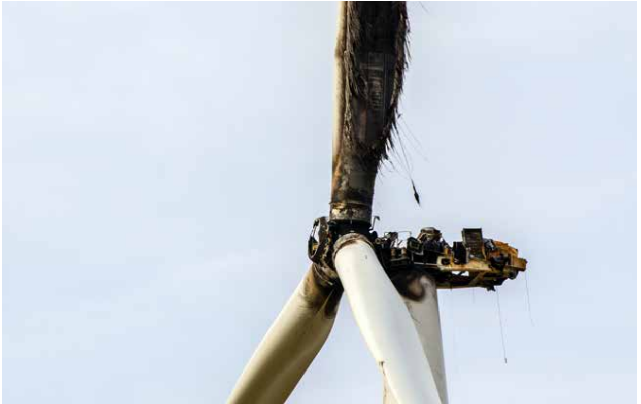
Some of the more common damage that lightning inflicts on turbines involves the blades. (Courtesy: Wojciech Wrzesien/Shutterstock.com)
