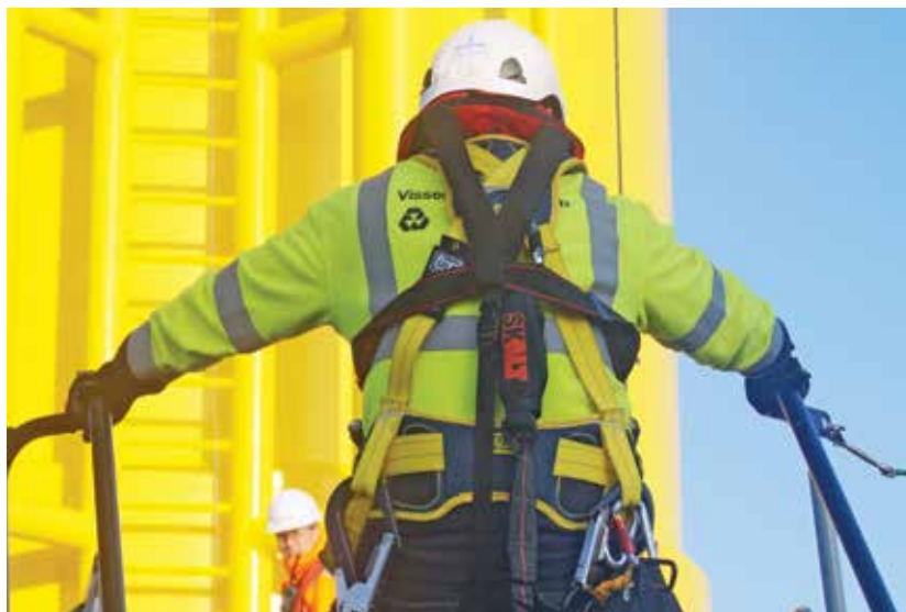
Visser & Smit Hanab employs one of the largest teams of in-house offshore wind specialists in the industry. (Courtesy: Visser & Smit Hanab)
