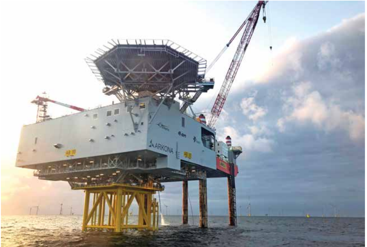
The electrical substation at the Arkona offshore wind farm is fully automated and is designed to be able to manage the wind farm autonomously. (Courtesy: Chantiers de l'Atlantique)
