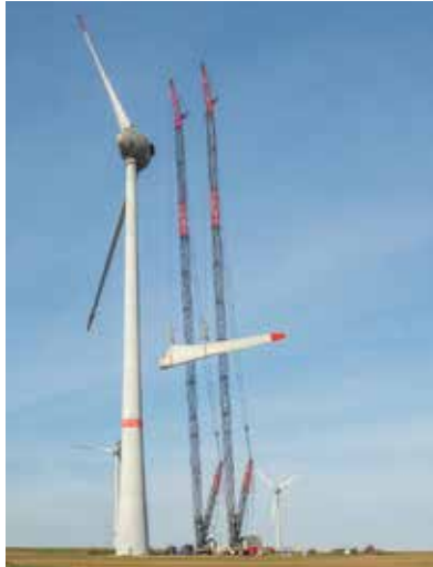
The 72-metric-ton, 58-meter-long rotor blades from an Enercon E-126 wind turbine at a height of approximately 136 meters are removed for maintenance. (Courtesy: Aertssen)
