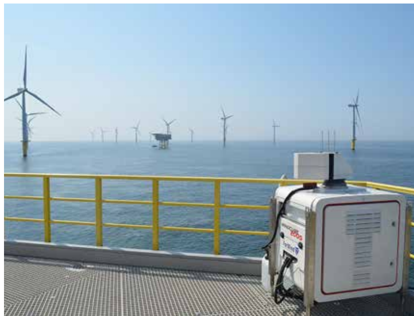
Stationary LIDAR measuring buoys deliver meteorological data continuously. (Courtesy: Fraunhofer IWES/© Jörg Schneemann, ForWind - Uni Oldenburg)
