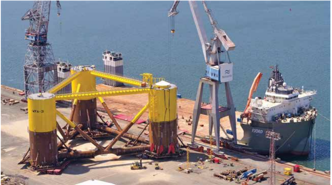
Construction and assembly of the more than 2,000-metric-ton structure took place as planned at the Navantia-Fene shipyard. (Courtesy: ALE)
