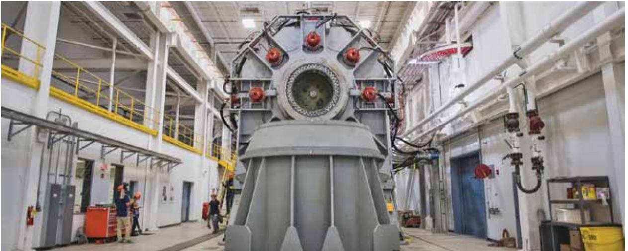
The test bed at the wind-turbine drivetrain testing facility. (Courtesy: Clemson)
