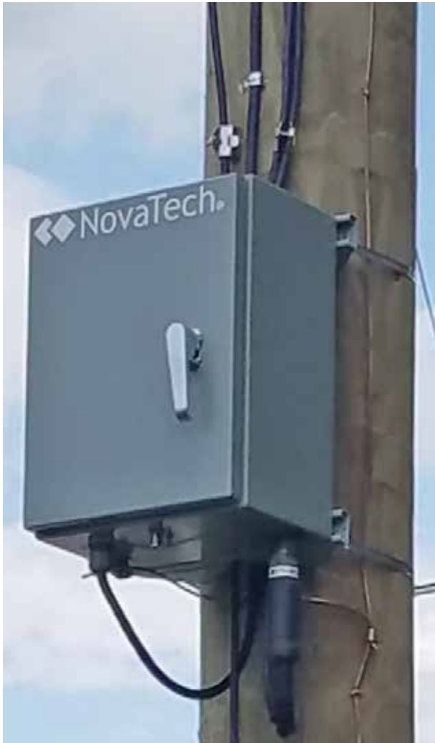
A DGM is a pole-top measurement system. (Courtesy: NovaTech)
