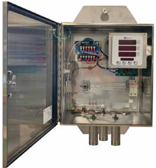
Three raw voltages and currents can be wired to a Bitronics distribution grid monitor (DGM). (Courtesy: NovaTech)
