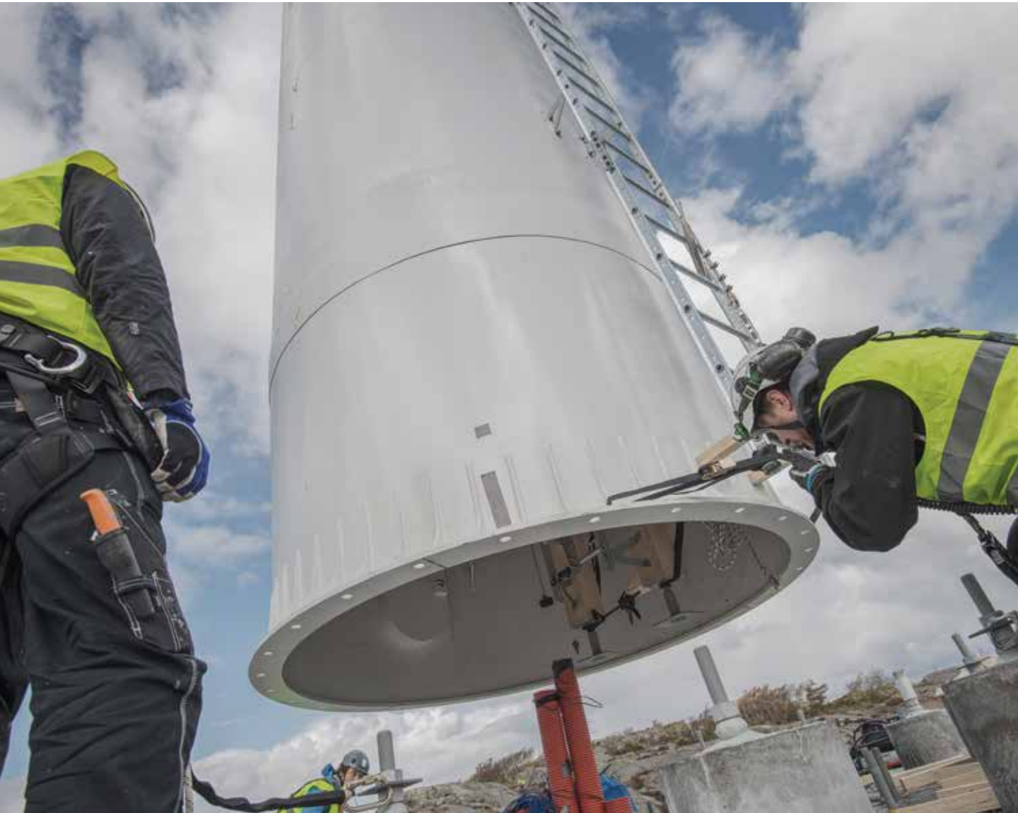
The first wooden towers will be built on a commercial scale by 2022. (Courtesy: Modvion)
