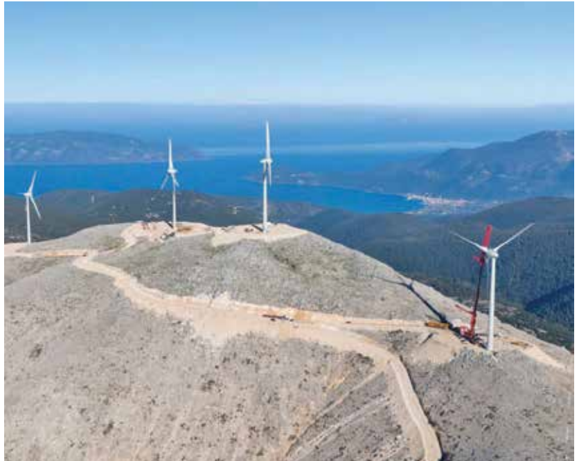
Ameresco's 9.2-MW Wind Project for PPC Renewables completes construction in Kefalonia, Greece. (Courtesy: Ameresco)
