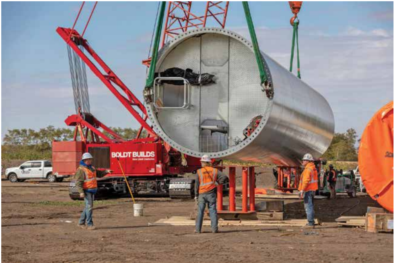
The towers, hubs, and blades were delivered and assembled at the base of the tower. (Courtesy: Boldt)
