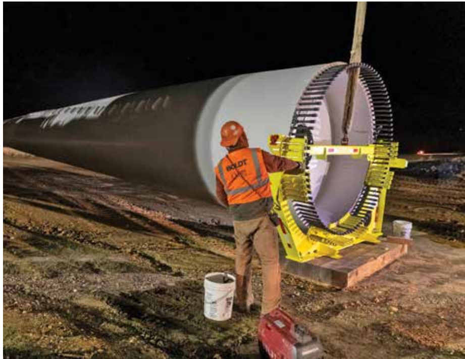
Night work is not unusual in the power industry, but when the jobsite is in the middle of a farm field, it's a new set of problems. (Courtesy: Boldt)
