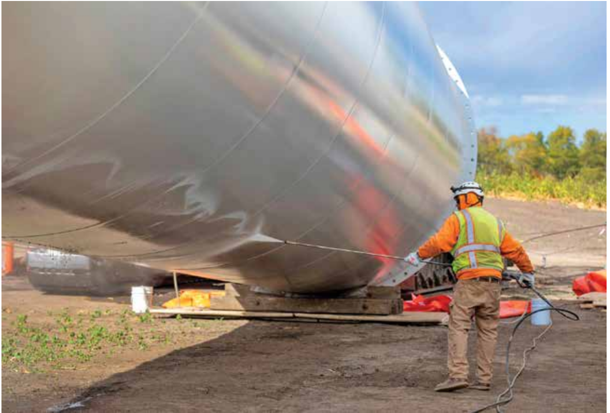
While the Boldt Company has been building wind farms since the early 2000s across the United States, construction of the Lone Tree Wind Farm presented a few unusual challenges. (Courtesy: Boldt)
