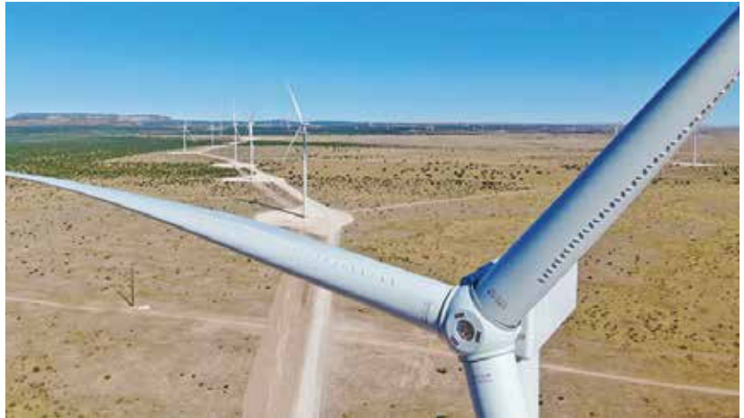
The four wind-power facilities that comprise Western Spirit Wind use a total of 377 GE wind turbines ranging from 2.3 to 2.8 MW in size. (Courtesy: Pattern Energy)
