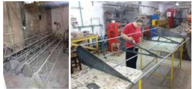
Figure 8: Turbine towers (left) and blade (right) after applying the protective zinc coat.
