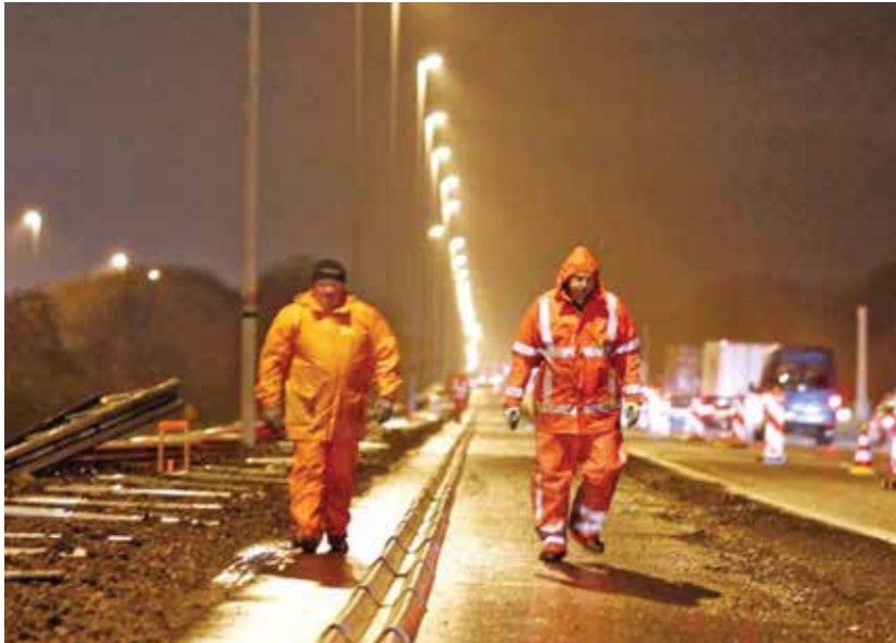
Pronomar systems can be helpful for workers in winter conditions. (Courtesy: Pronomar)
