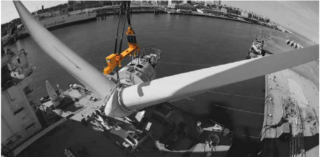
With Airpes' expertise being mostly focused on wind energy, its specialized equipment has been fitted to work with Crosby's hardware to complete onshore and offshore installations. (Courtesy: Crosby)
