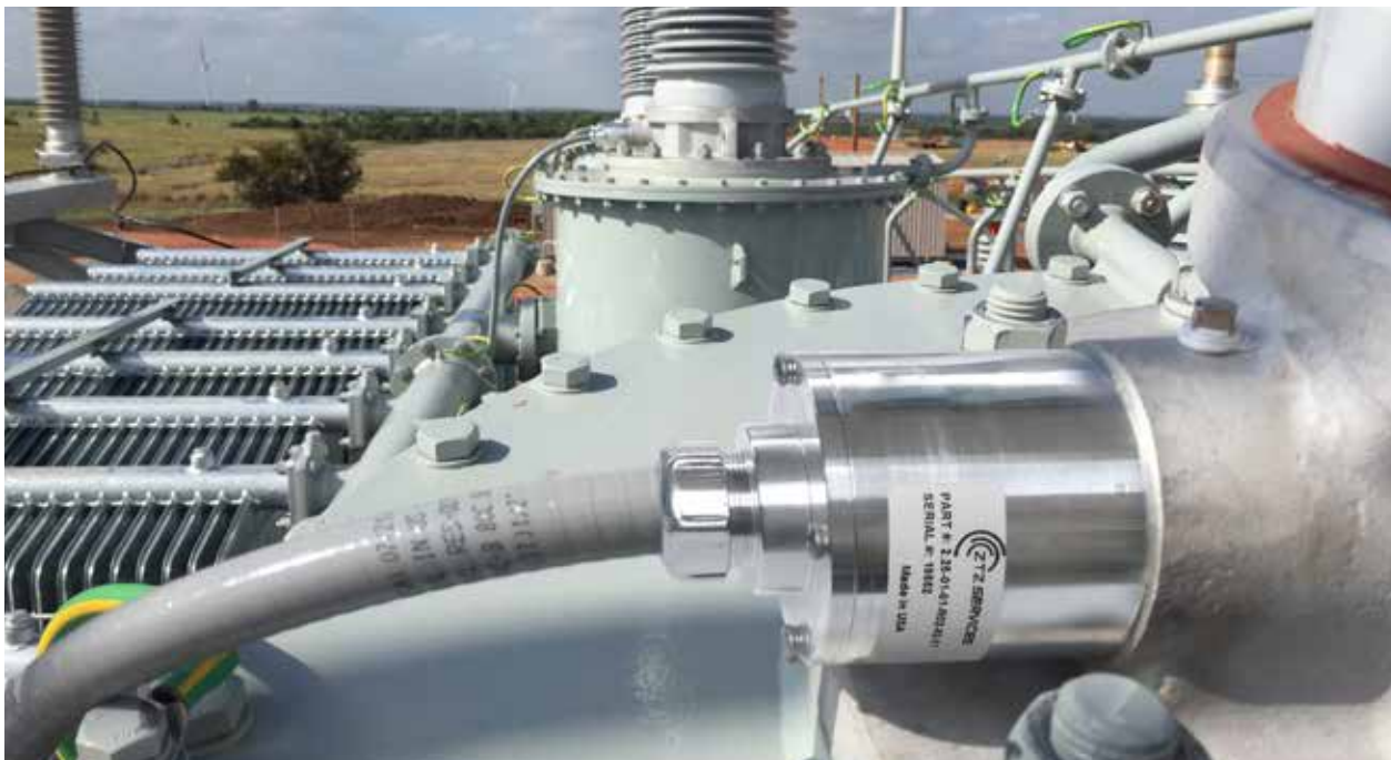
Three bushing sensors on the main step up transformer at Walla Walla Washington NextEra Site. (Courtesy: ZTZ Services International)
