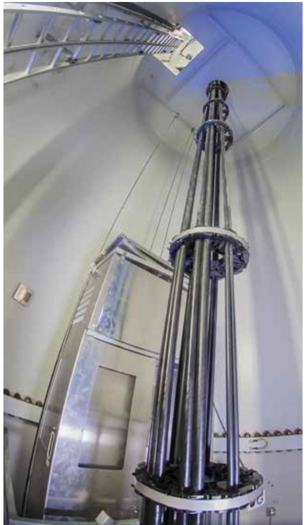
Top and above: The cables replaced during an overhaul can vary based on what equipment is being upgraded or repaired. With thousands of components in an entire turbine, a majority of the cables replaced are in the nacelle and the drip loop, where cables experience millions of torsion cycles over their lifespan. (Courtesy: Helukabel)
