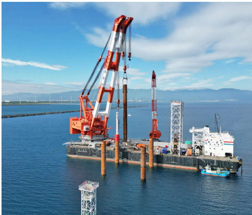
Full construction begins on Ishikari Offshore Wind with first installation of an 8 MW offshore wind turbine in Japan. (Courtesy: Pattern Energy)
