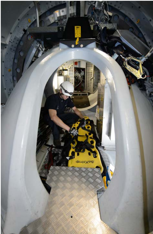
A technician demonstrates proper use of life-saving rescue equipment in a real-life setting. (Courtesy: Wind Academy by Siemens Gamesa)
