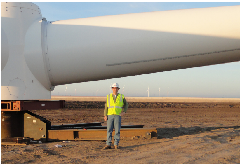
ArcVera’s CEO and Principal Atmospheric Scientist, Gregory Poulos, at a wind-farm construction in progress. The ArcVera technical leadership team prefers to engage directly in work in progress, traveling to project sites as the technical scope of work requires. (Courtesy: ArcVera Renewables)
