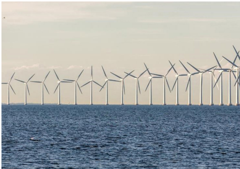
An offshore wind farm project supported by Bureau Veritas. The organization supports both onshore and offshore wind projects, leveraging dedicated solutions for blades, gearboxes, generators, towers, and foundations for both. (Courtesy: Bureau Veritas)
