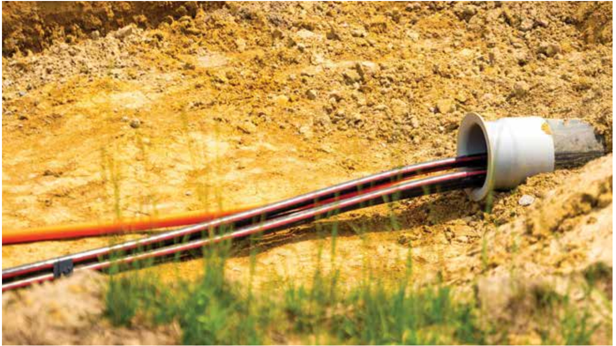
Medium-voltage underground distribution cable allows for the low-loss transport of electric power generated by wind-collector arrays. (Courtesy: AWG)
