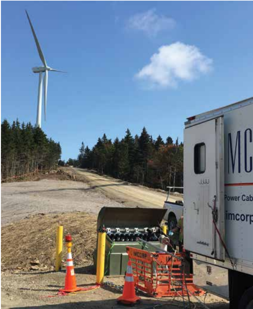
Good installation practices of accessories play as important of a role in long-term cable reliability. (Courtesy: AWG)
