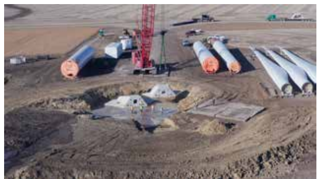
Photo 2: Pre-cast concrete sections are lifted into position at the Palmers Creek Wind Farm in Granite Falls, Minnesota. The sections will be post-tensioned and then backfilled before tower erection begins. (Courtesy: Barr Engineering Co.)
