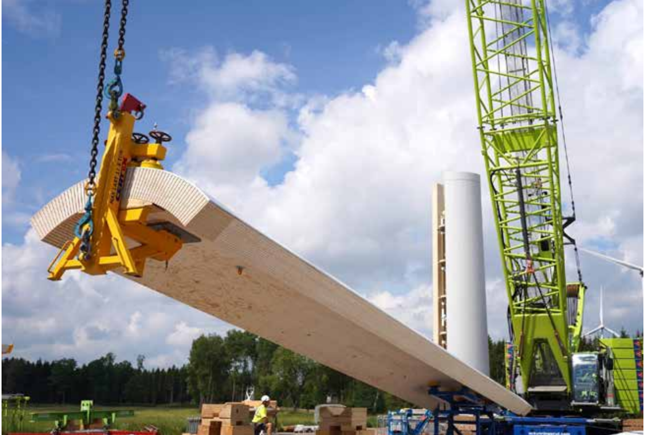
The wood technology company Modvion is building a 105-meter wind-turbine tower made of wood, the tallest of its kind, in Sweden. (Courtesy: Modvion)
