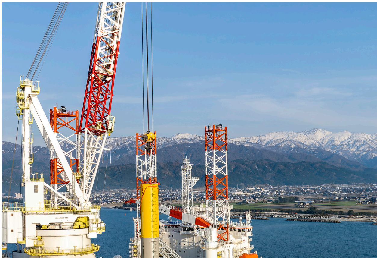
FOWIC will, in corporation with Shimizu, make use of the jack-up vessel Blue Wind for the project. (Courtesy: Fred. Olsen Windcarrier)
