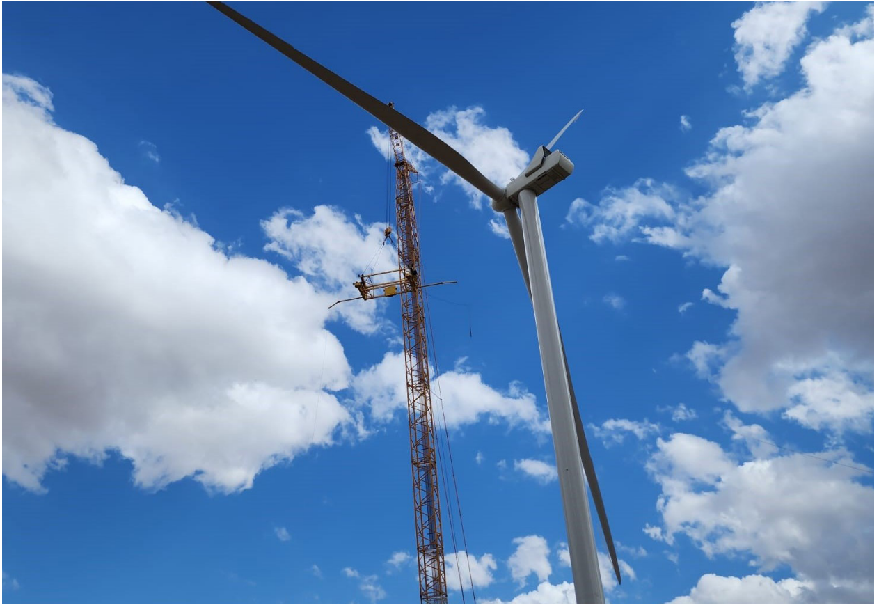
The Whitla Wind facility has an installed capacity of 352.8 MW, which allows it to generate enough energy to power more than 100,000 homes per year. (Courtesy: Sarens)
