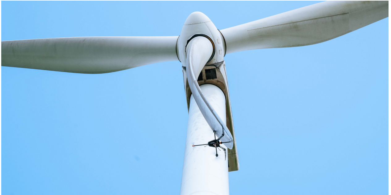
A Voliro T drone inspects the lightning protection system of a wind turbine in Indonesia. (Courtesy: Indonesia Suprabakti)
