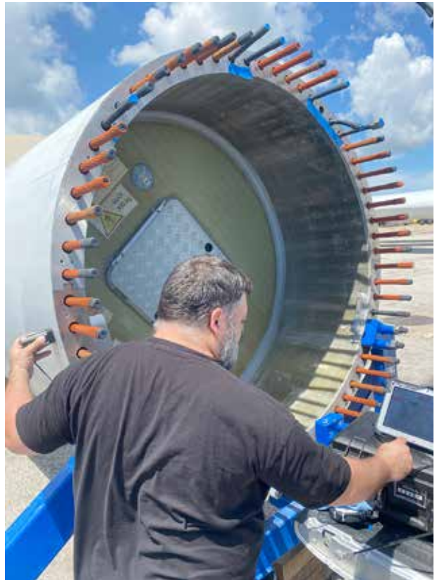
One of the most dangerous risks to a wind turbine is under-torqued bolts at the root connection. (Courtesy: CICNDT)
