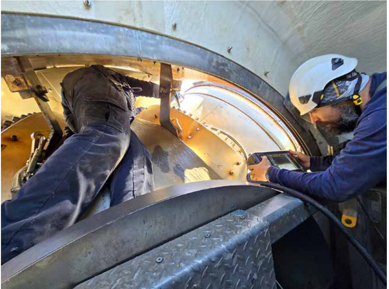
Maintenance teams face a constantly evolving list of risks: leading edge erosion from rain and sand, lightning strike damage, temperature-induced fatigue cracking, and progressive weakening of adhesive bondlines. (Courtesy: CICNDT)
