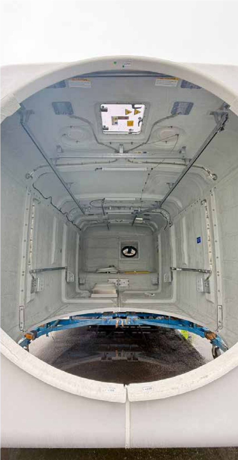
A nacelle cover protects the gearbox, generator, and electronics inside from wind gusts, lightning strikes, salt spray, and thermal cycles. (Courtesy: BlueWind)
