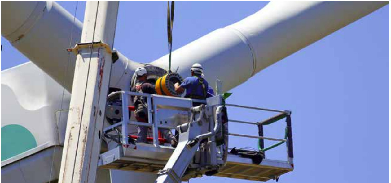
Wind turbine technician roles require a blend of technical training and physical skills. (Courtesy: Shutterstock)
