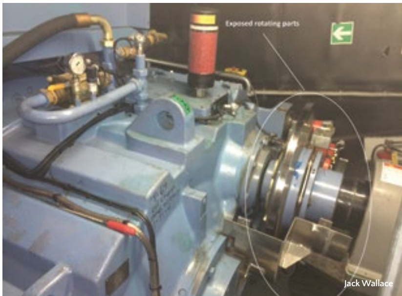
The dangers of moving objects illustrated by a gearbox with an exposed brake disc and high-speed shaft
