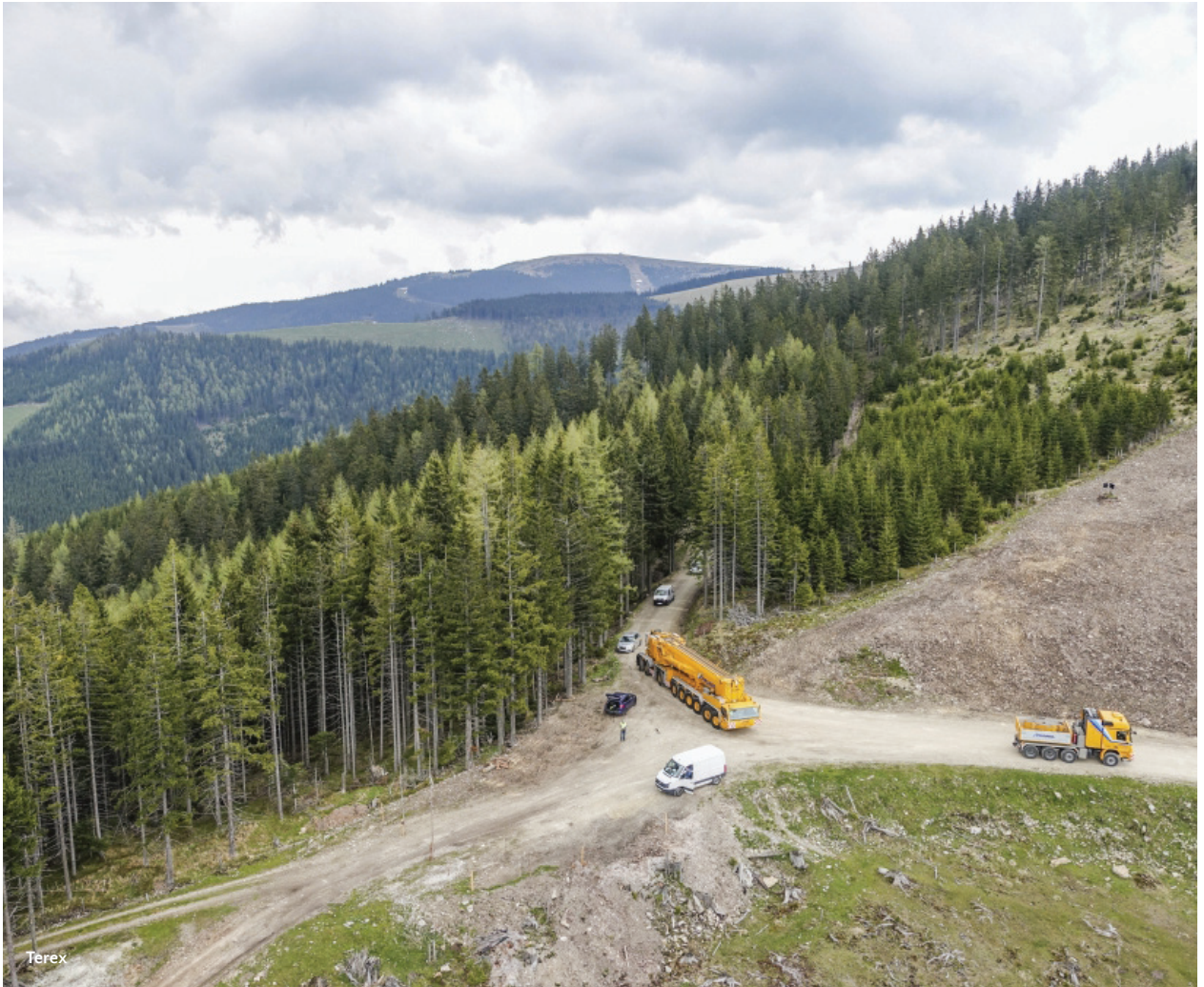
The AC 1000 All Terrain Crane drives to the top of the Pretul.
