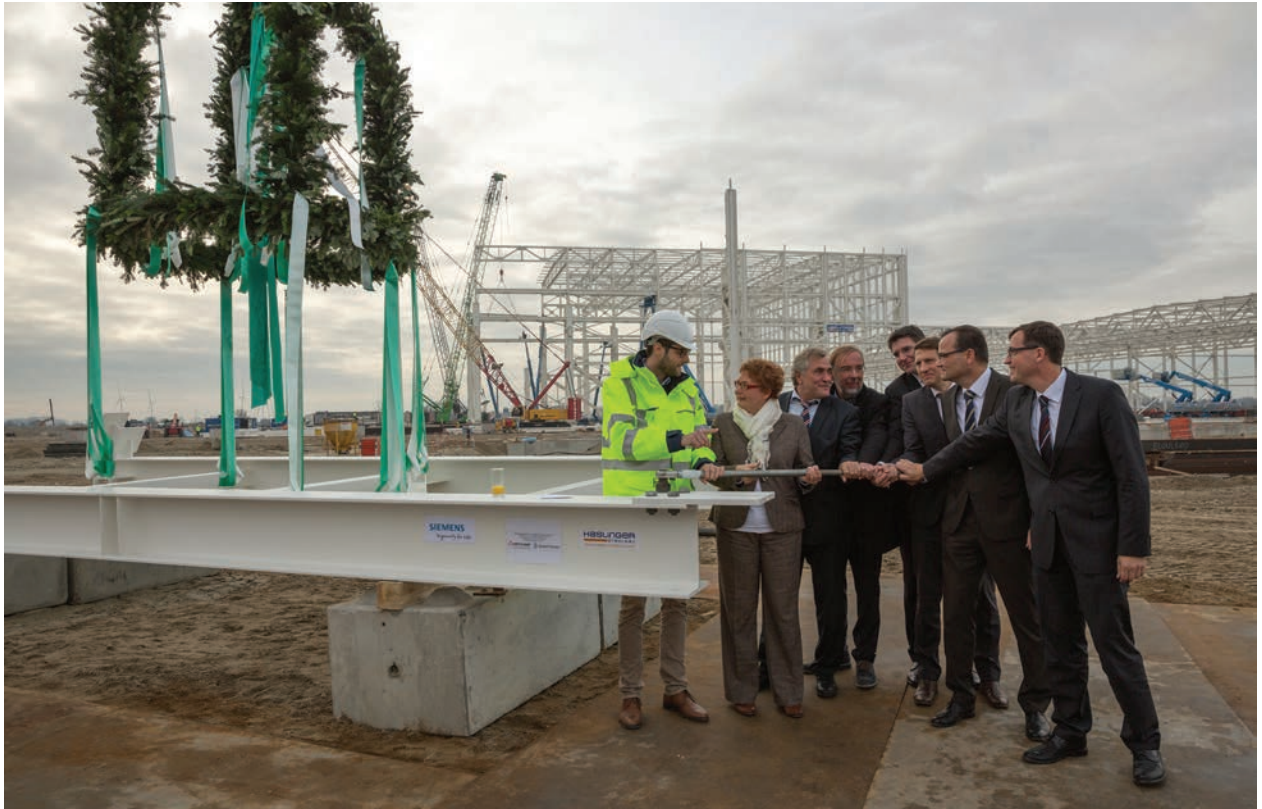
Siemens celebrates the topping-out ceremony for its new wind-turbine manufacturing facility in Cuxhaven, Germany. Julian Egger, on the left in the safety equipment, is tightening a steel pin together with the political leaders and company representatives. (Courtesy: Siemens)
