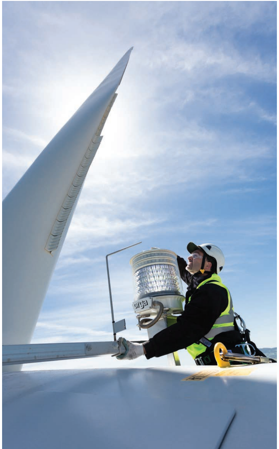
Siemens provides service and maintenance for more than 4,000 installed wind turbines in the Americas region. (Courtesy: Siemens)
