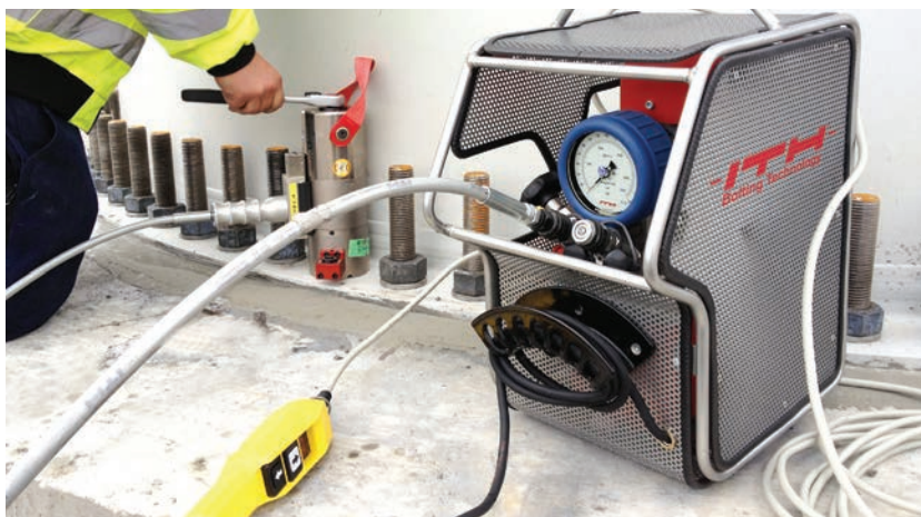
ITH performs wind-turbine bolting services on-site all over North America — also from its sub-offices in Atlanta, Georgia, and Houston, Texas. Above, wind-turbine foundation bolts are tightened precisely by an ITH bolt tensioning cylinder type MS and a compact high pressure pump unit Micro-MAX 70.
