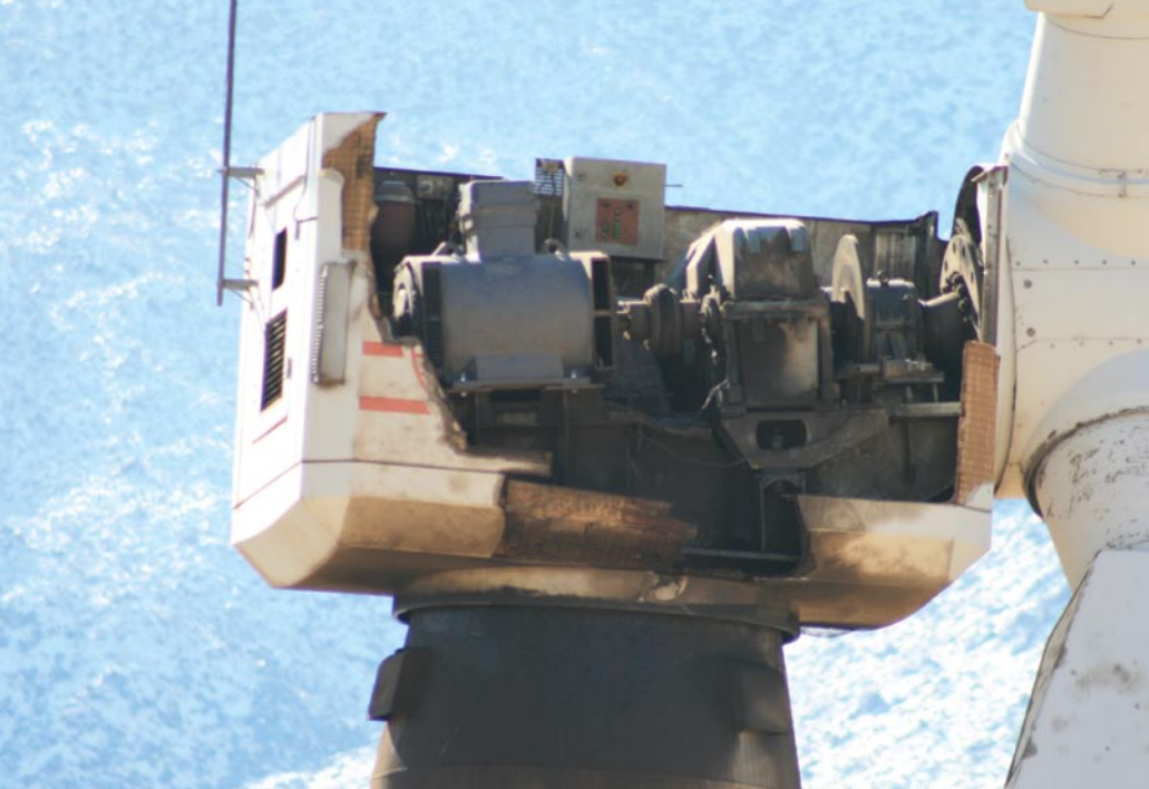
Fig. 3: The aftermath of a turbine fire.
