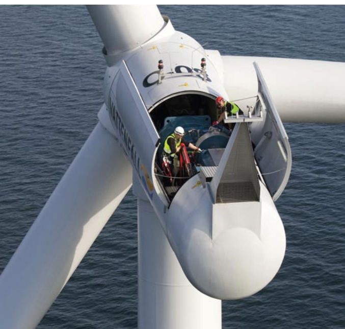
Fig. 7: Close-up of the rotor hub and opened gondola of a wind turbine at the Swedish offshore wind farm Lillgrund, type SWT-2.3-93 with a rating of 2.3 megawatts (MW).
