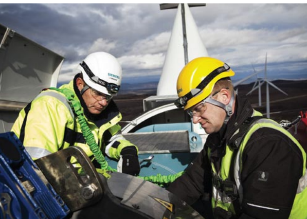
Fig. 6: Siemens service technicians at work on a SWT-2.3-82 at Farr Wind farm in Scotland. The 92 MW farm is owned by npower renewables and is comprised of 40 Siemens SWT-2.3-82 turbines.
