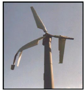
Fig. 2: Lightning caused catastrophic blade damage.
