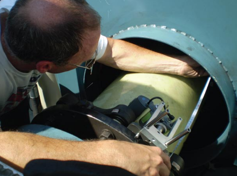
Fig. 2: Pre-alignment duties involve taking off the coupling guard, and in some cases installing a turning gear and a rotor lock so brake will remain disengaged.
