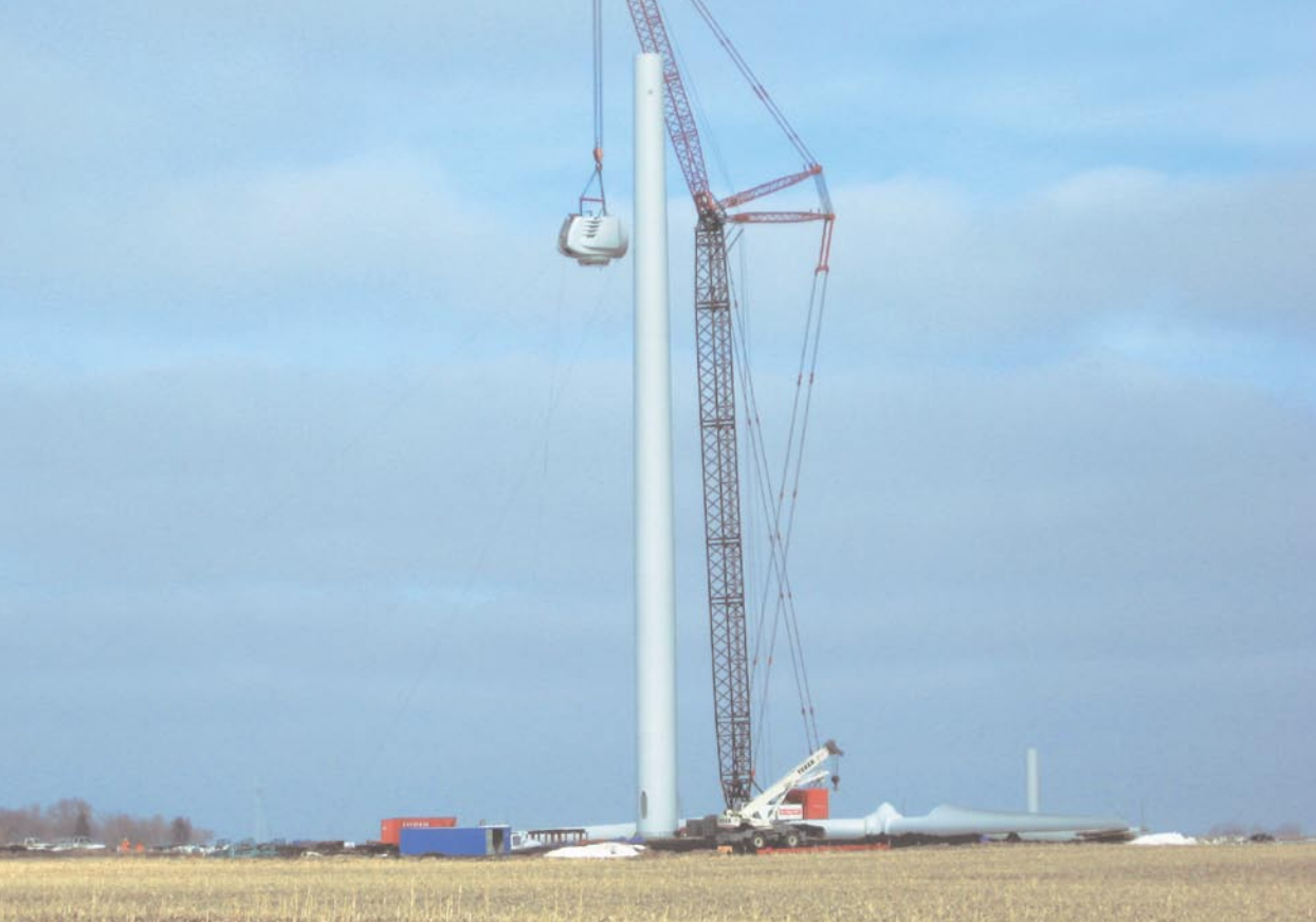
Fig. 4: A nacelle is lifted into place at the Endeavor Wind Energy Center.
