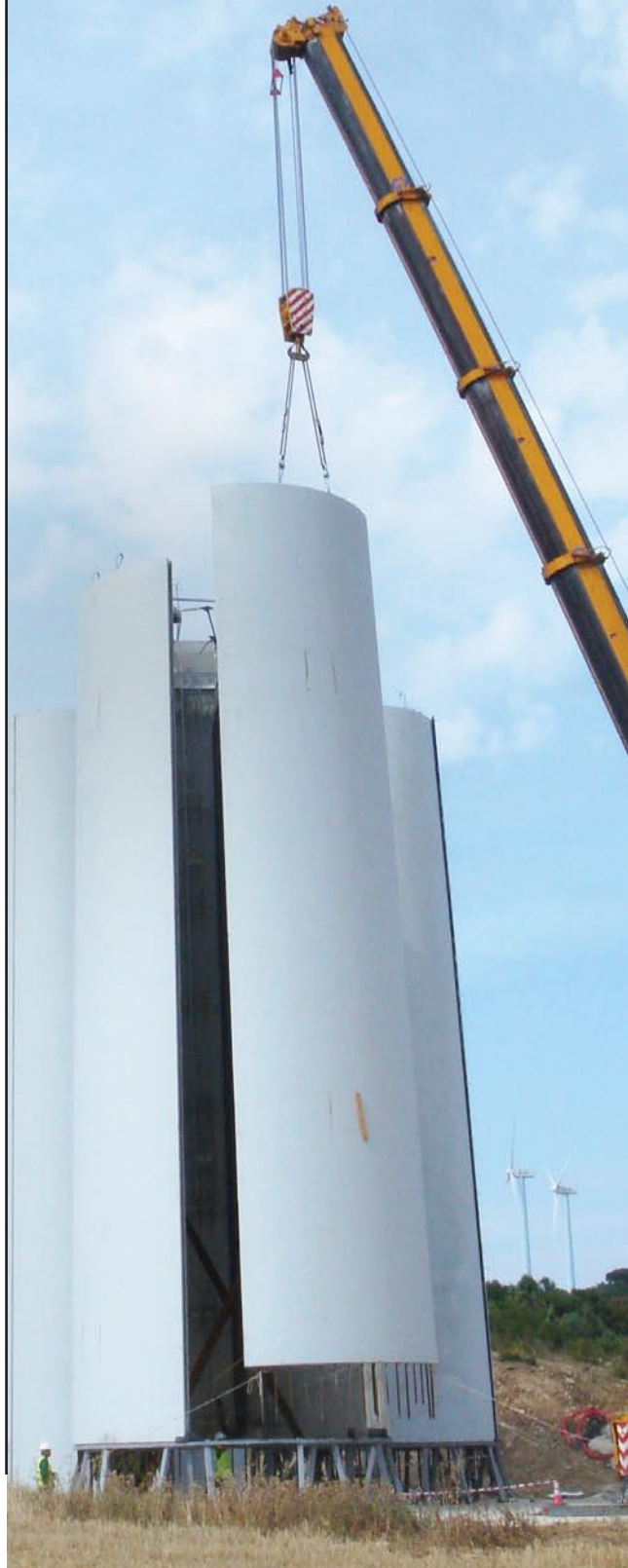
Fig. 4: More pre-assembly operations at the Peñablanca Wind Farm, featuring a tower of 100 m.
