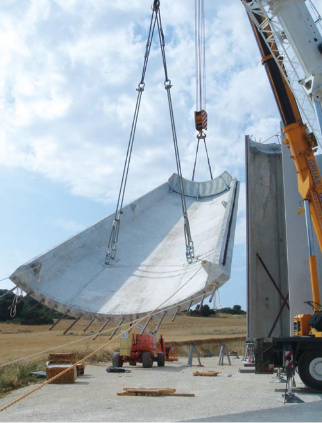
Fig. 2: The Peñablanca Wind Farm in Spain, where the patented preassembly process allows rates of more than two towers per week.
